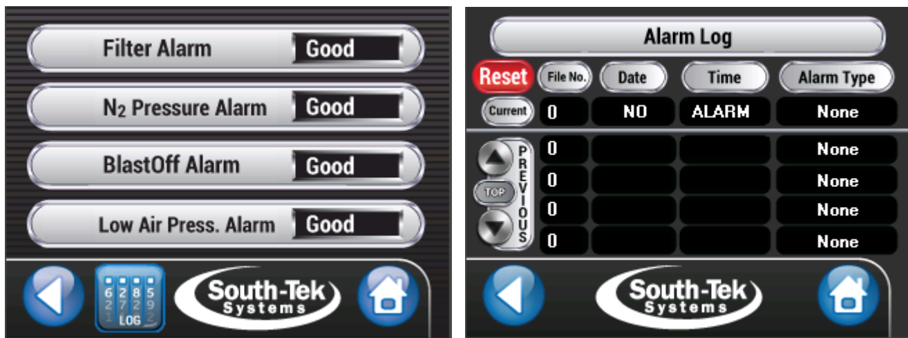
Figure 12: Alarm Screen(left) and Alarm Log(Right)
